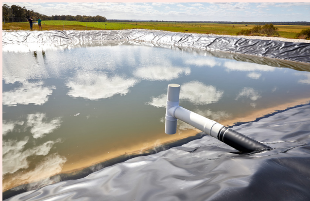
Primary solids sedimentation pond with T-piece transfer system.
