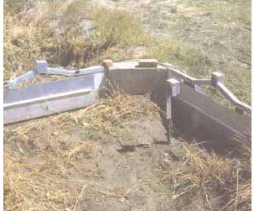
FIGURE 5.5 Electronic flood gates
