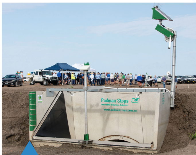
Padman automation fitted to infield infrastructure
