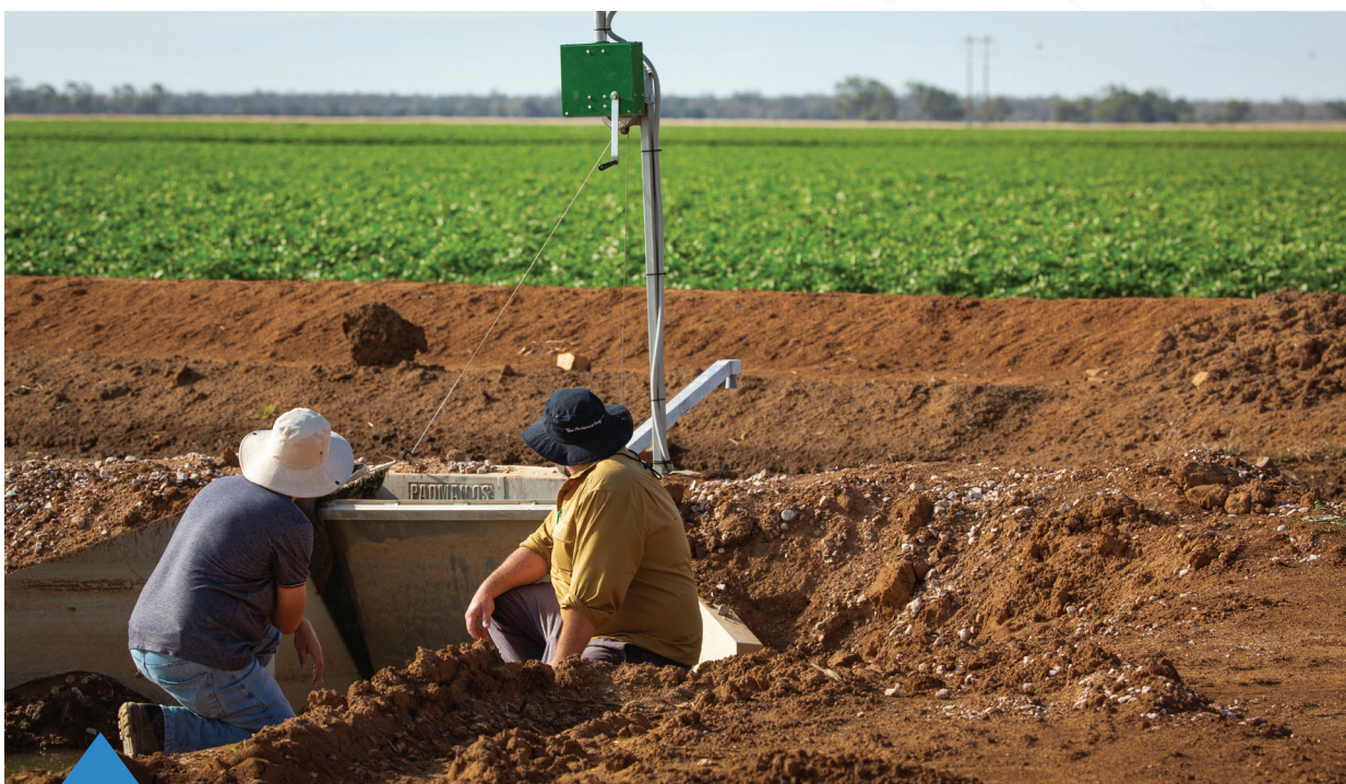
Example of automated Padman autowinch fitted to an inlet in field
