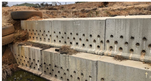
Weeping wall allows liquid to be separated from solids.
